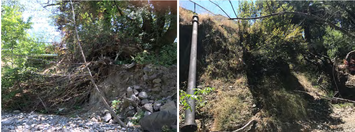
Active bank erosion on right bank of Sonoma Creek within the main campus.
