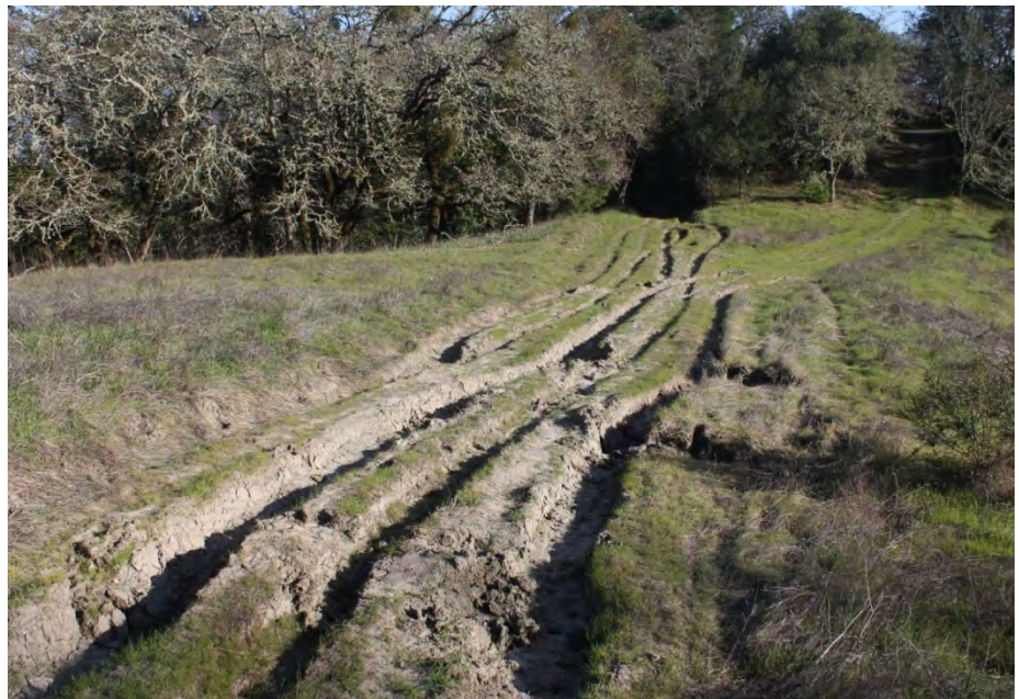
Deep ruts and erosion along an access road.
