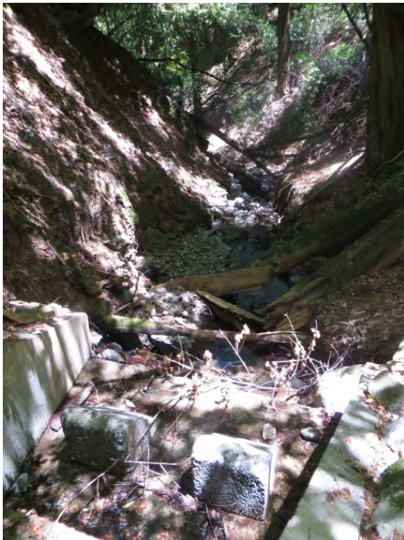
Looking downstream at culvert (top); looking downstream at baffles for energy dissipation (bottom)
