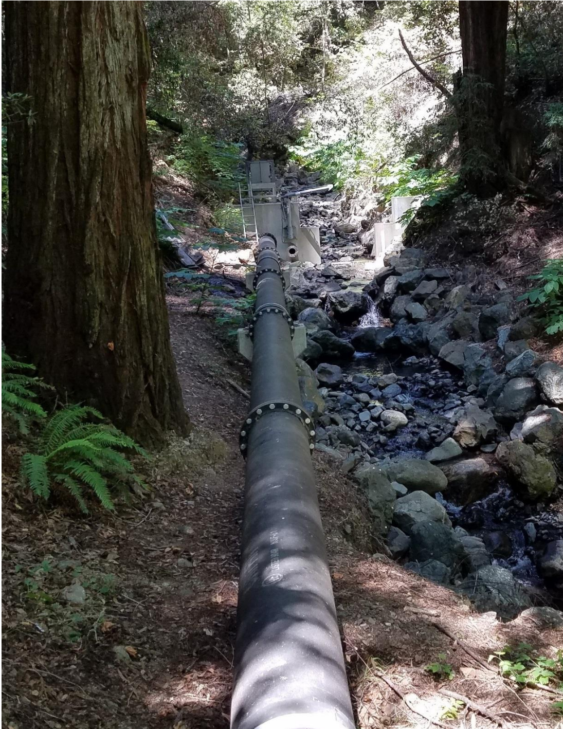
Photo 2: Asbury Diversion. Note the small pipe opening in the weir wall designed to allow 0.9 cfs stream flow to bypass diversion.
